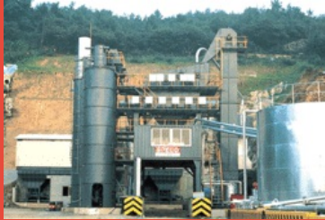
Speco Hot Mix Plant
